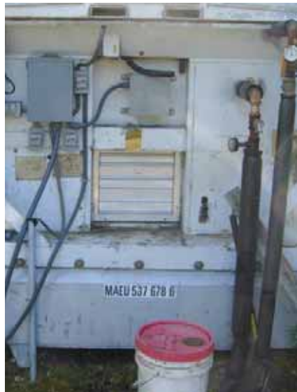
Kiln controls are located on the rear wall of the container.
